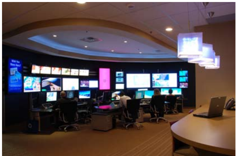
Diversified Media Group's control room manages a digital signage network in the Time Warner Center in New York City.
